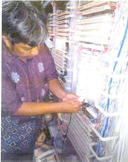
Gambar 3.4. Instalasi Server Call Center
